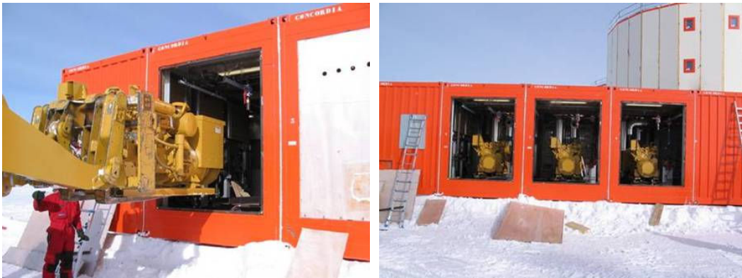
Fig. 6. A set of three 125kW diesel generators provide the electrical power for Concordia Station. (photos - IPEV)
